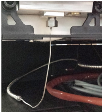
pressure sensor placed into the output hydraulic circuit
